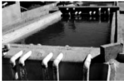
Washing water purification system
